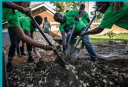
Building a ramp to increase accessibility at EmbraceKulture during group community service
